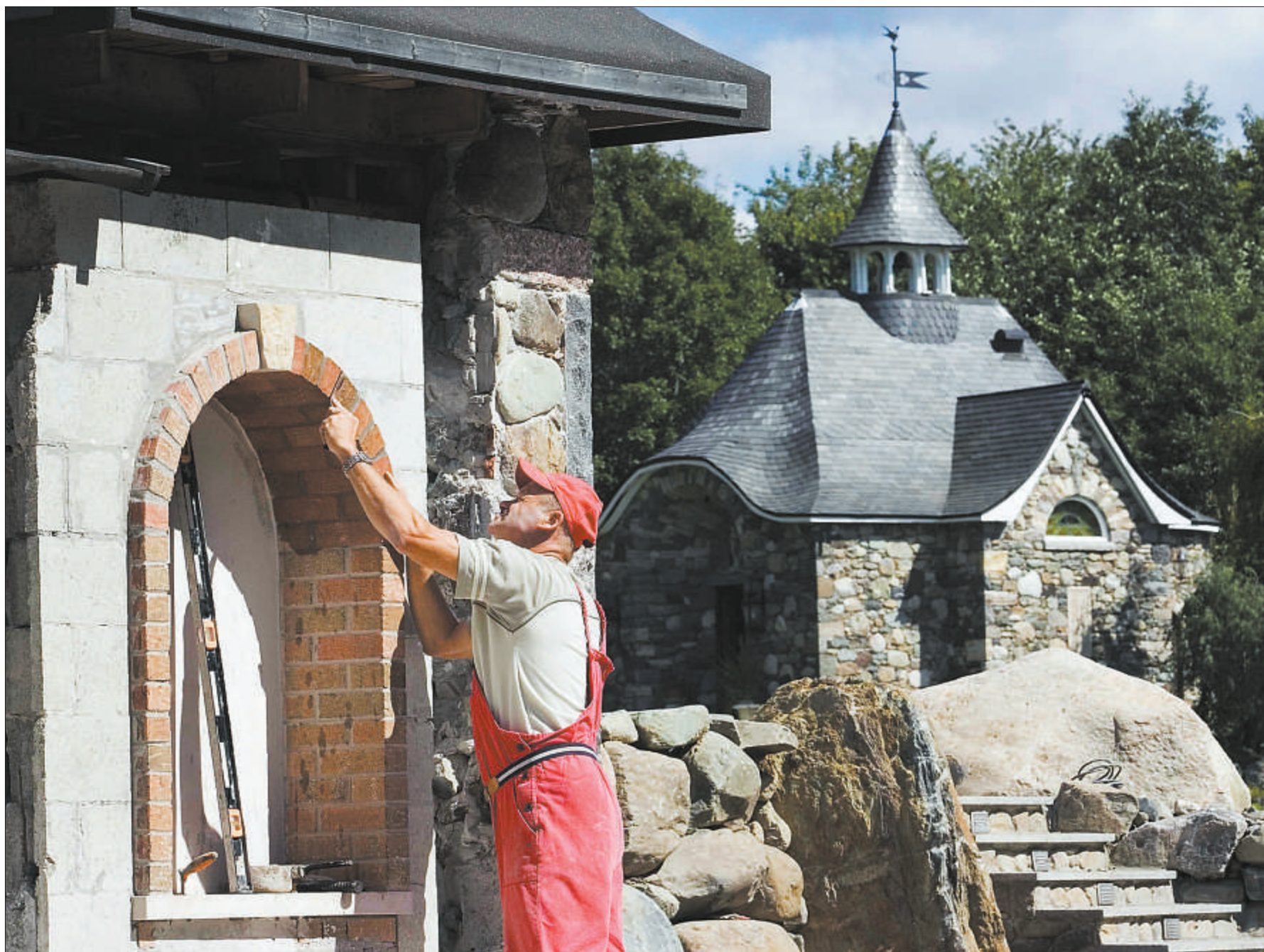
Master mason on the job: Czech craftsman Josef Mrkva is hard at work at Chapelle Ste. Agnès, a stunning estate of terraced vineyards and Old World architecture near Sutton. Mrkva and his son are specialists in vaulted ceilings, a kind of architecture that is standard in underground wine cellars in Europe but unknown here.
